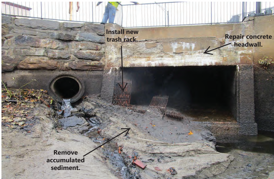
Photo 17: View north of the 24" RCP stormwater culvert and mill race box culvert. Note the deteriorated trash rack and accumulated sediment. 10/16/2022.
