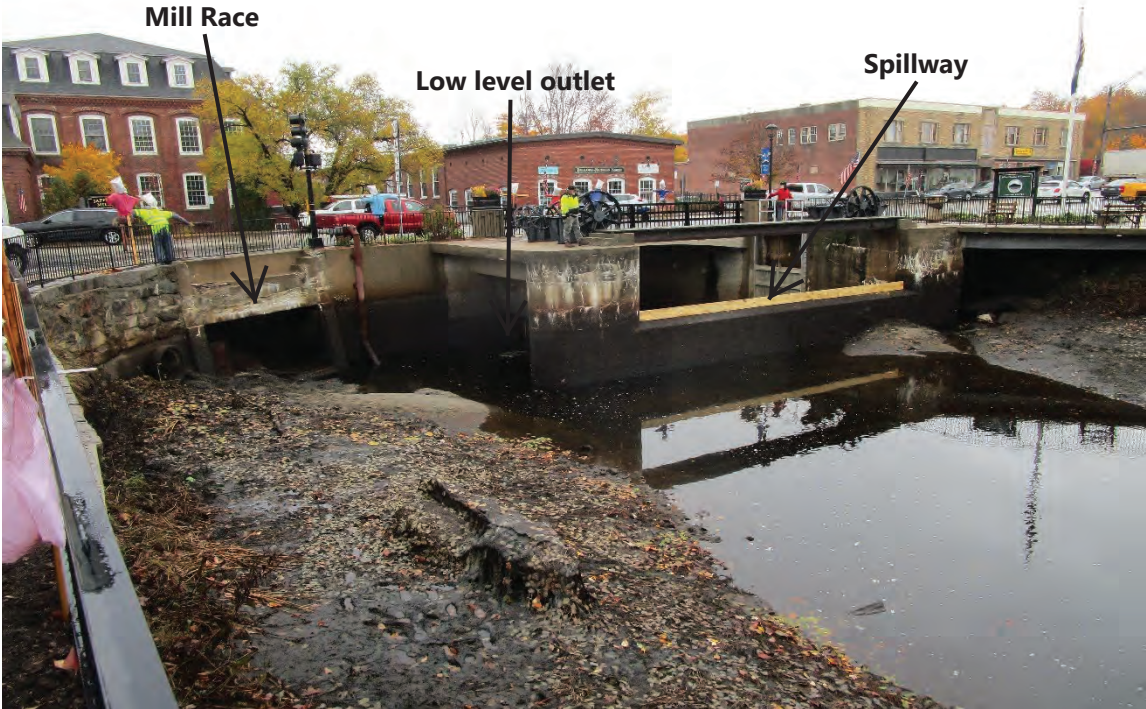
Photo 15: View northeast of the Site towards the existing Main Street Bridge during drawdown conditions. 10/16/2022.
