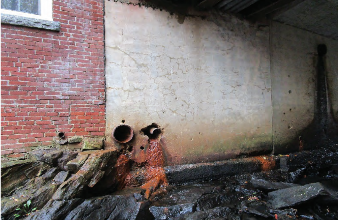
Photo 23: View southeast of the confluence of the Main Street Bridge with the mill building. Note the pipes present in the concrete bridge wall. 10/16/2022.
