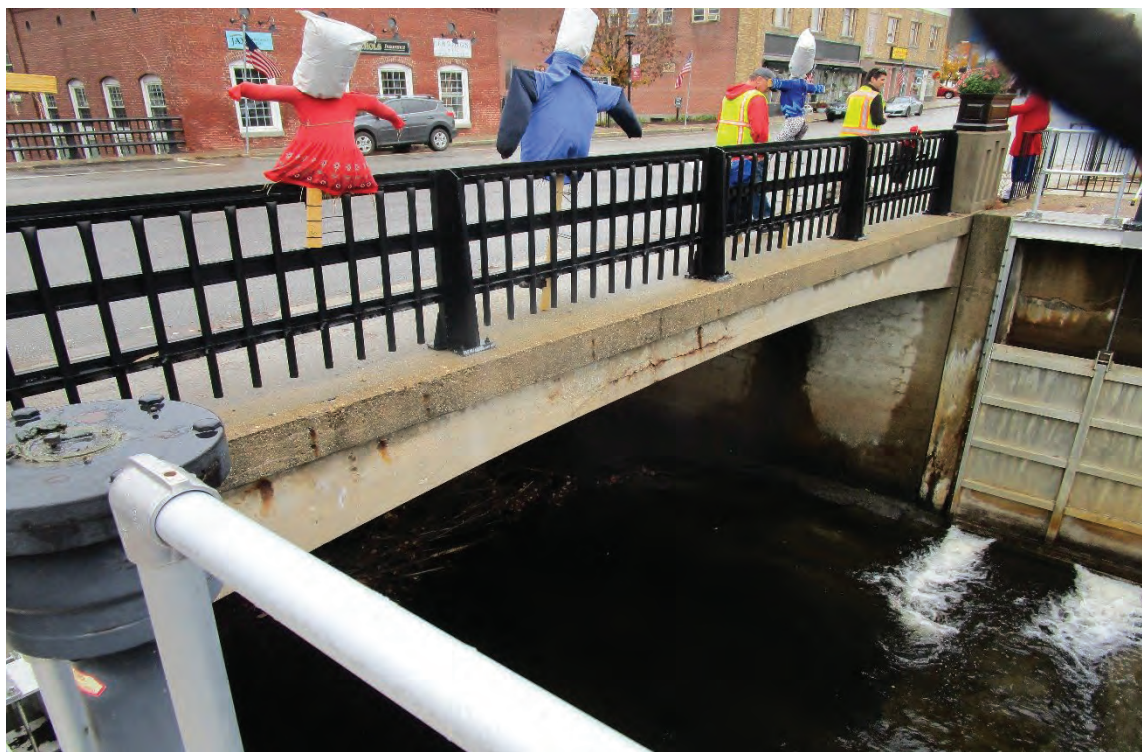
Photo 18: View east of the concrete damage along the sidewalk on the existing Main Street Bridge. 10/16/2022.
