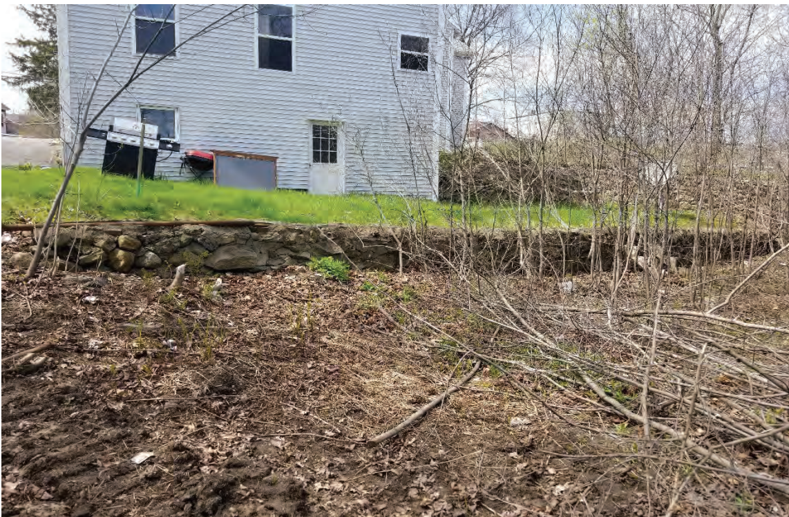
Photo 26: View northwest of the retaining wall on NHDOT Parcel #11 taken from near the top of bank of the river. 05/05/2022.
