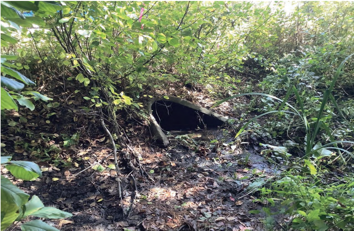
Photo 4: View northeast of the culvert within the depressional scrub-shrub portion of Wetland 1. 10/07/2021.
