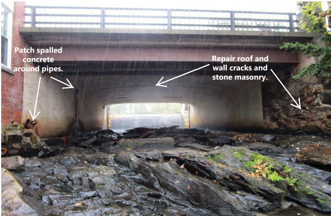
Photo 21: View southwest/upstream of the existing Main Street Bridge with the spillway visible in the background. 10/16/2022.
